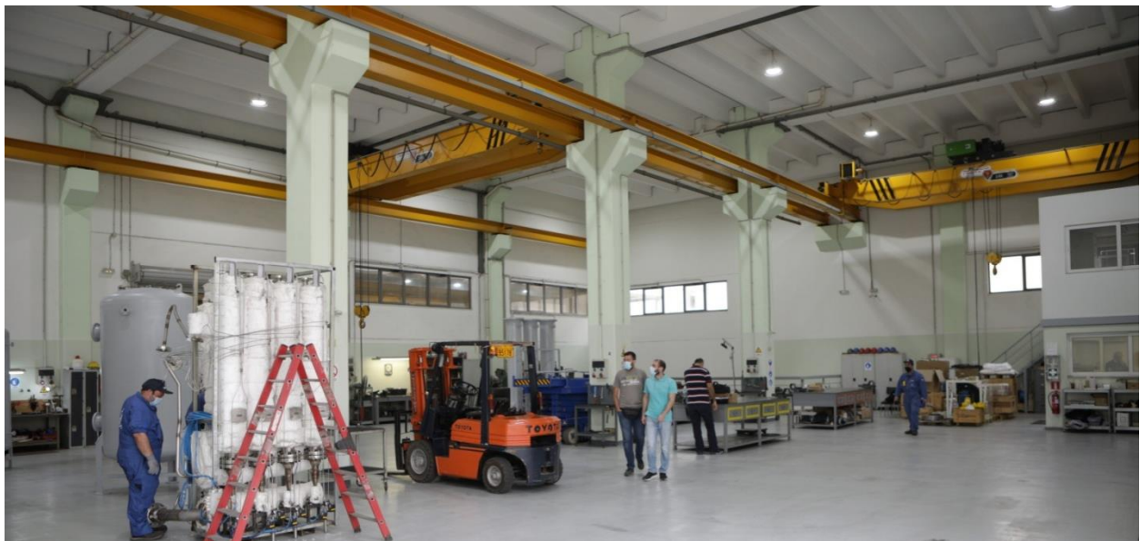
The construction of the Hydrogen Generator at the premises of Carell S.A. in Perama, Greece.
